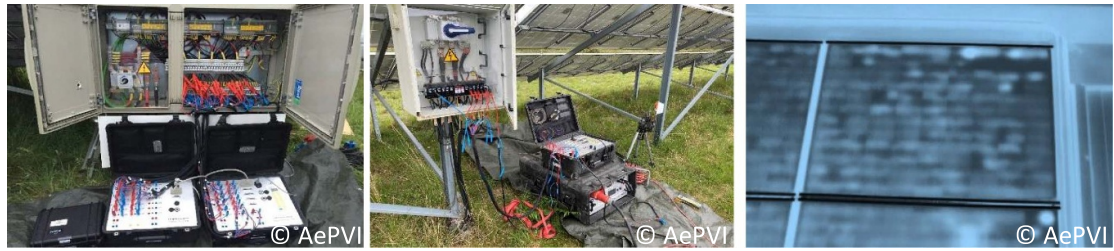
Figure 9. Equipment used for energizing the PV strings at a combiner box (left and center), IR_{INV} image recording of a PV module revealing cell breakage (right).
